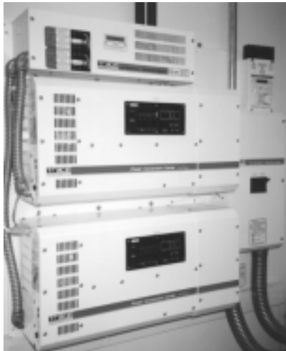
Dual 4 kW Trace sine wave inverters to provide 120 and 240-volt AC power from a 48-volt DC battery bank
