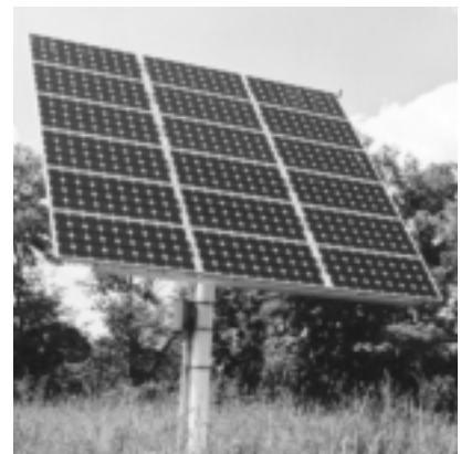
Pole-mounted solar PV array on motorized tracking mount
