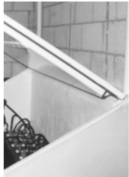
Site-built insulated battery box. Note the gasketed lid and rear PVC pipe vent to outside.
